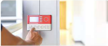
FIRE & BURGLAR ALARM SYSTEMS
