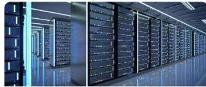
DATA SERVER IMPLEMENTATION
